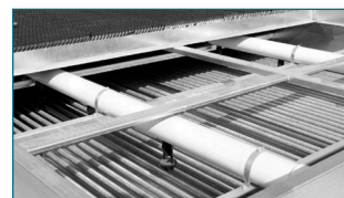
Drift Eliminators Removed for Coil Inspection
