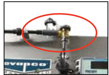
Figure 6 – Conductivity Probe and Flow Switch
