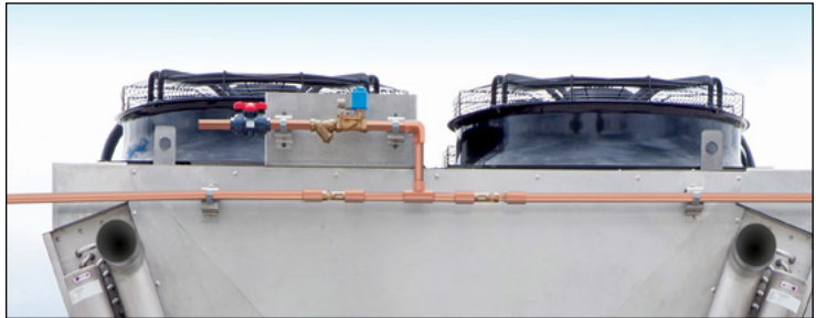
Water supply solenoid valve arrangement
