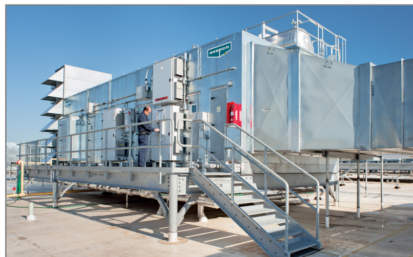
Critical Process Air (CPA) Hygienic Air Handling System
