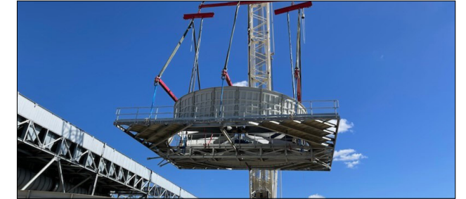
Advanced Technology™ ACC Onsite Modularization
