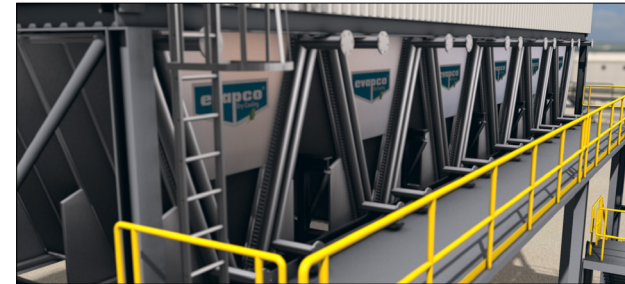
eco-Air Titan™ Multiple air cooled heat exchangers (ACHE) Tube Bundles Positioned Beneath Large Fans
