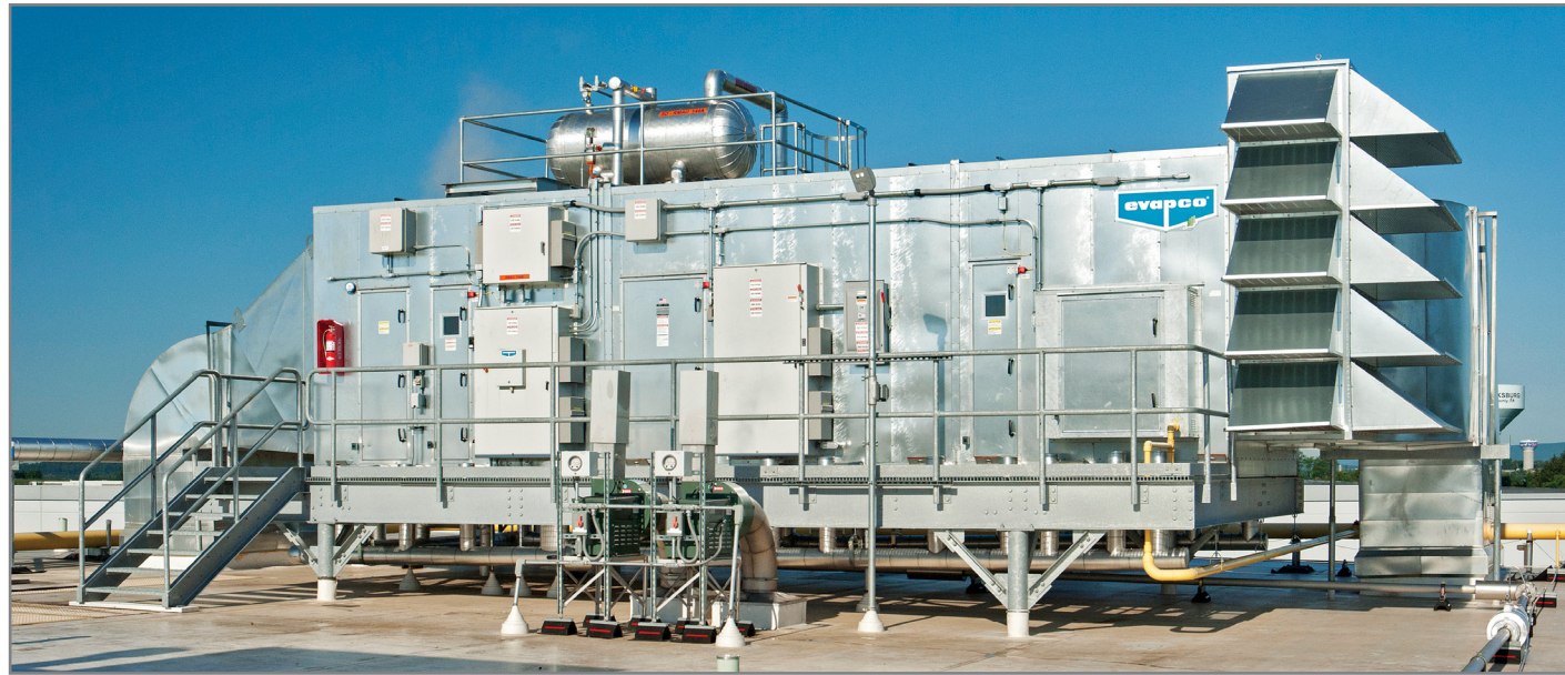
Critical Process Air (CPA) Hygienic Air Handling System
