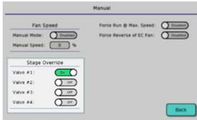
Manual Valve Opening Enabled
