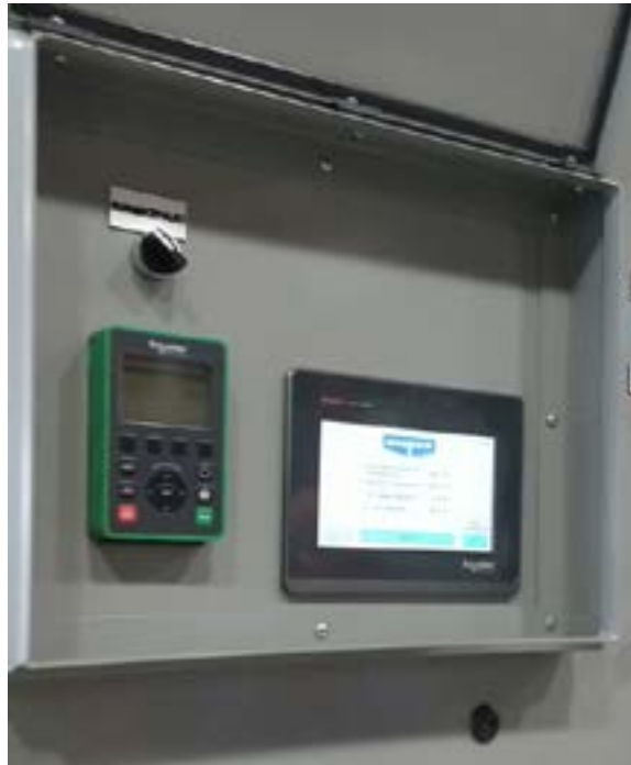
HMI, VFD and Bypass/ Off/Auto Switch for NEMA Motors
