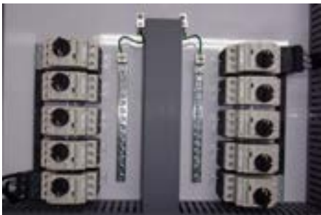
MMP in Control Panel
