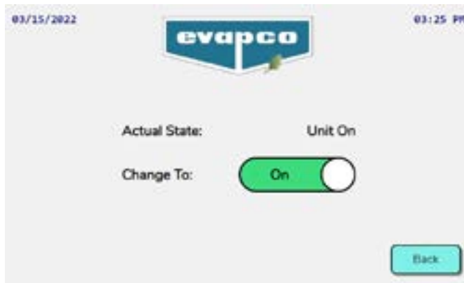
eco-Air Unit Turned On Locally
