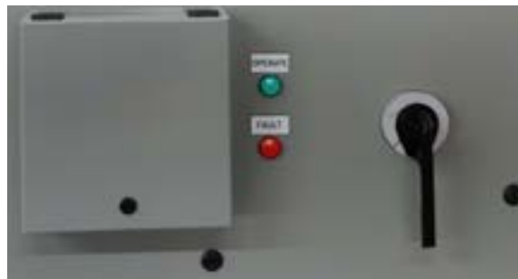
Main Disconnect in OFF Position
