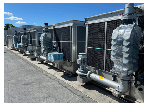
Figure 5: Smart Shield™ Chemical Feeders on Condensers Awaiting Shipment.
