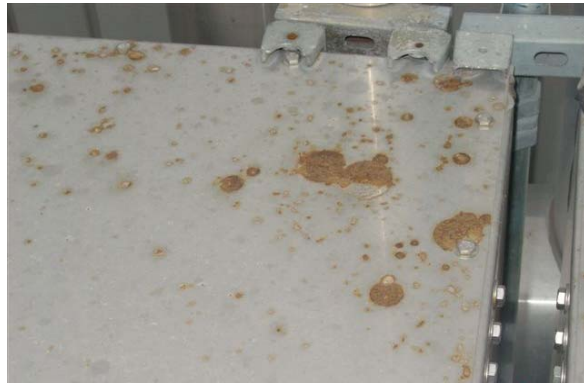
Unit located at a textile plant (Weld Spatter)
