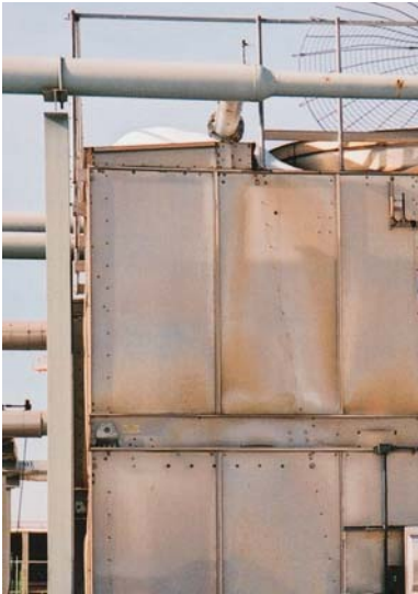
Unit located next to an airport (Atmospheric Corrosion)
