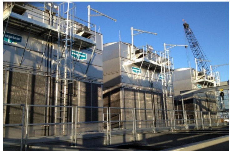
Figure 2 – Stainless steel cooling towers
