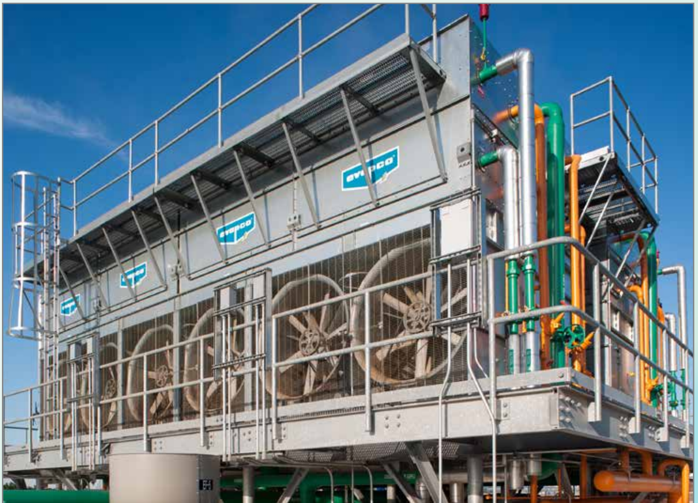
PMC-E Evaporative Condenser with external service platform.
