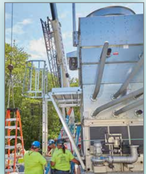
eco-ATWB-H Closed Circuit Cooler installation
