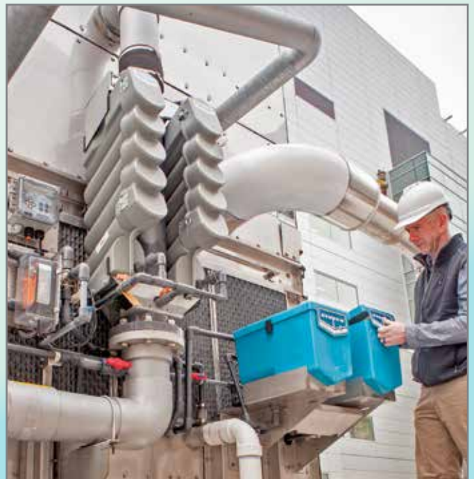
Smart Shield® Factory-Mounted Water Treatment System
