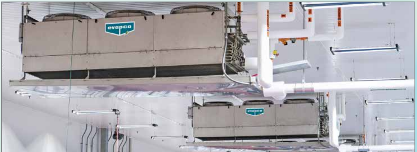
SSTWE Work-Room Evaporators
