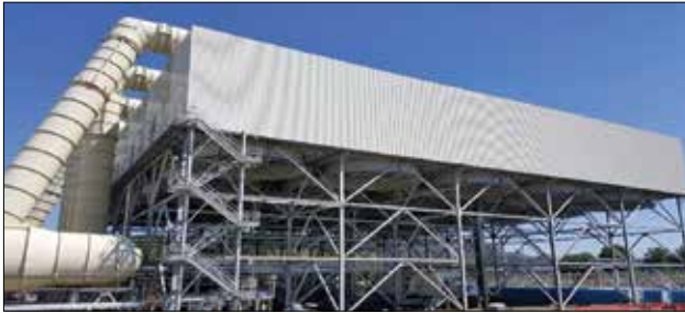
Two condensers, one structure
