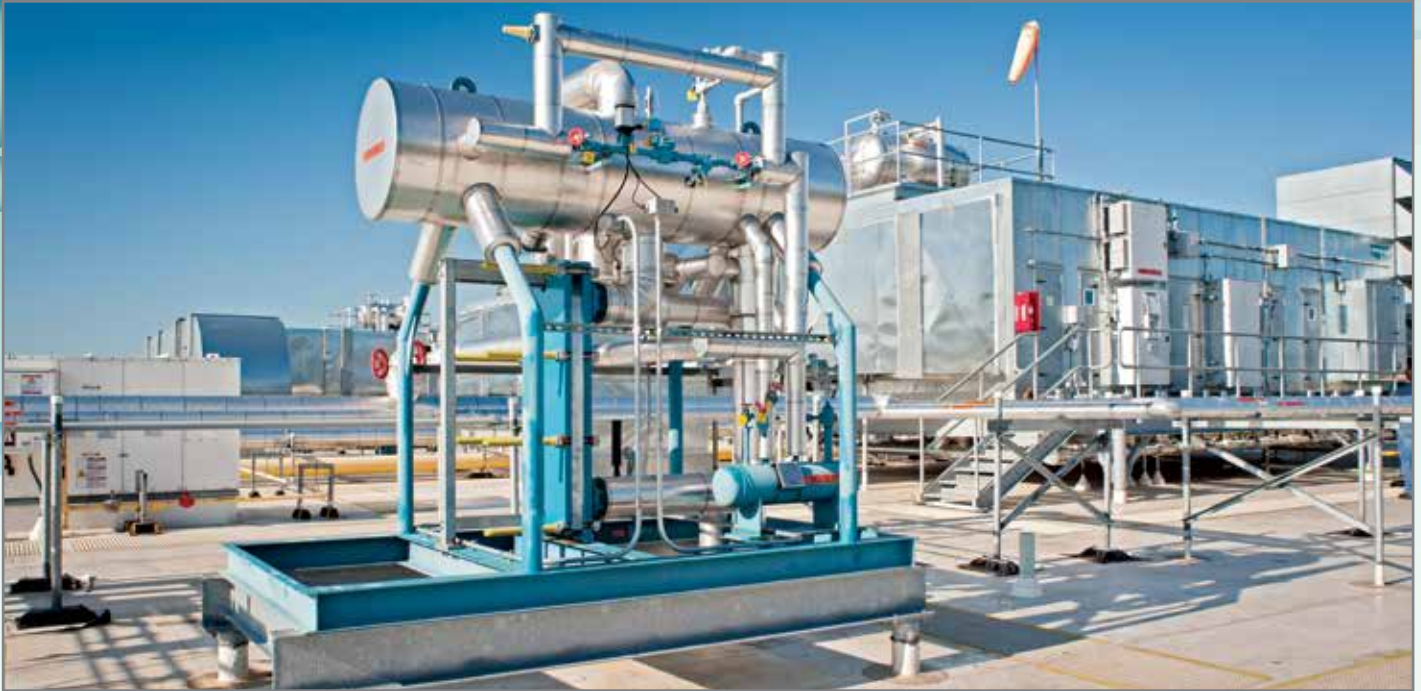
RVS MPC Chiller Package
