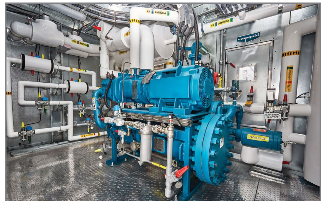
Evapcold Low Charge Ammonia Machinery Room LCR-P-W
