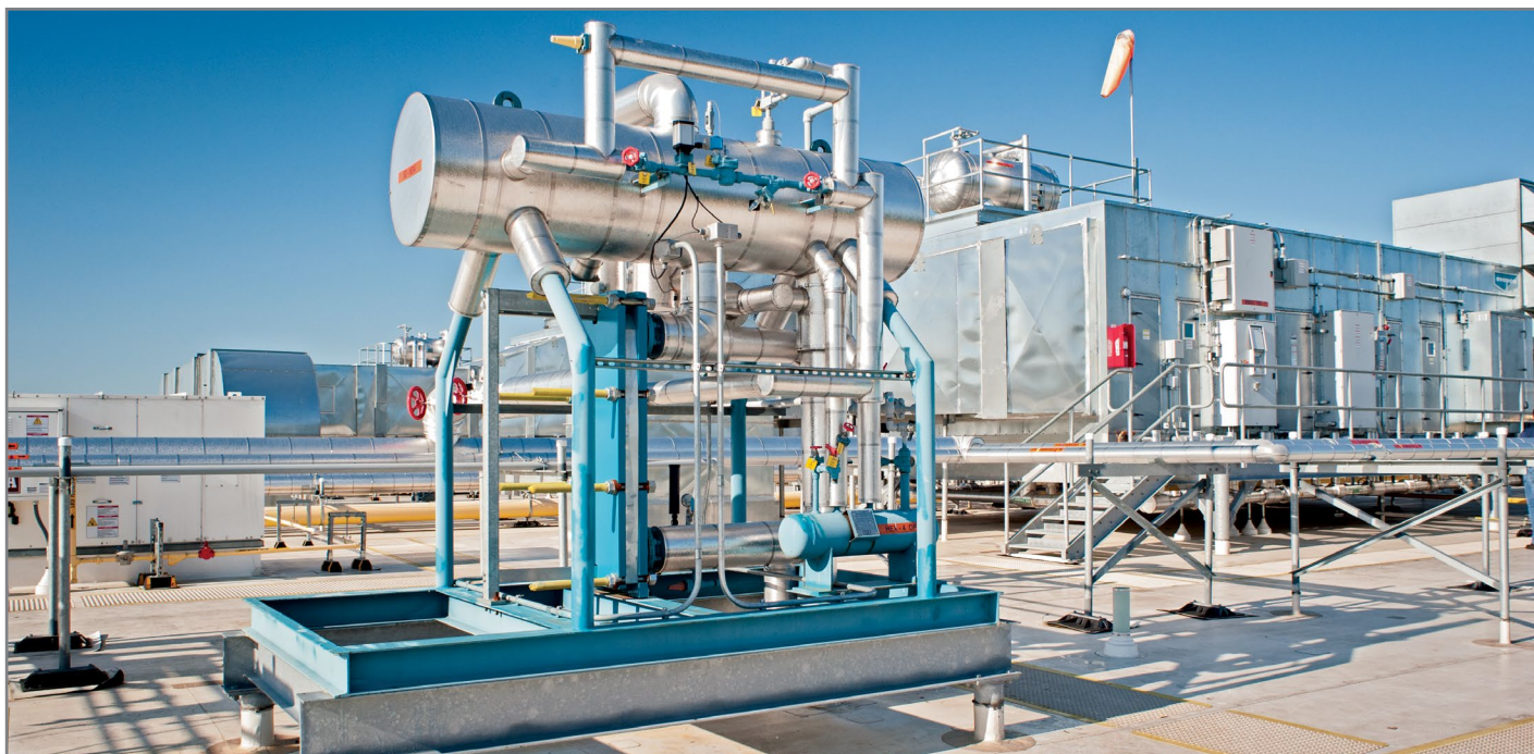
RVS MPC Chiller Package
