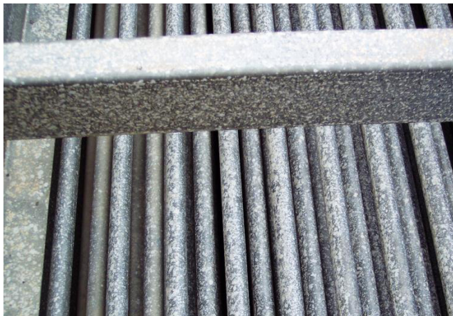
Figure 1: Evaporative Condenser With White Rust
